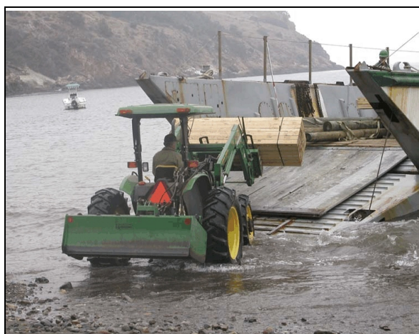
Figure 4. Unloading hacking tower construction materials from a NPS landing craft at Prisoner's Harbor, Santa Cruz Island, California.
